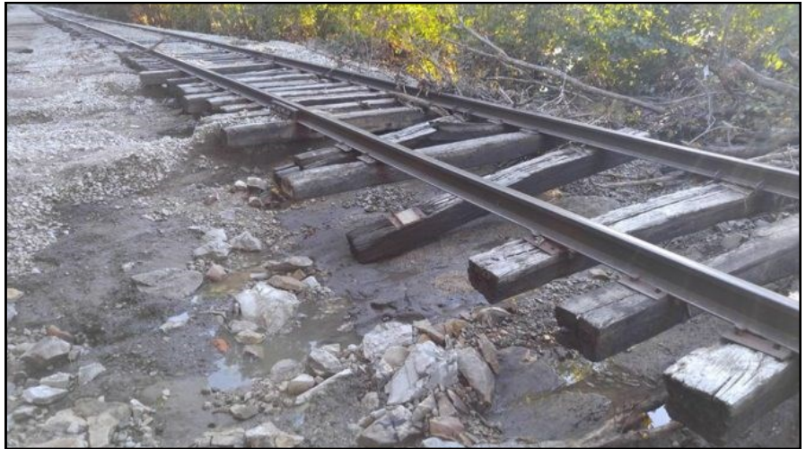
Figure 1: Washed out railroad tracks near Ottawa, Kansas. Picture via MidlandRailway.org
