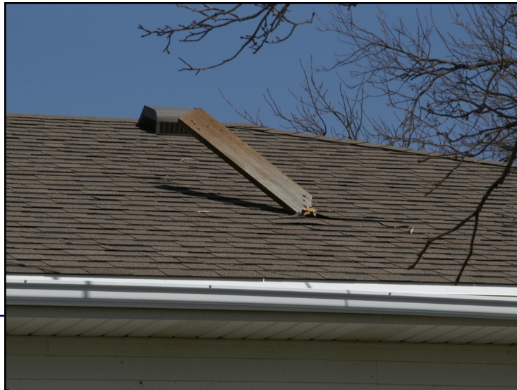
A piece of debris impaled the roof of a house as a result of strong winds associated with a weak tornado in Nemaha County the evening of March 23rd. Photo by Ken Harding, used with permission.
