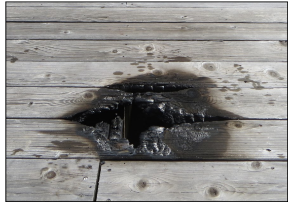
Lincoln, Montana at Krohn Lake, June 24-25, 2014. Photo by Janet Sholder. Cabin deck was burned/ melted after being struck by lightning.
