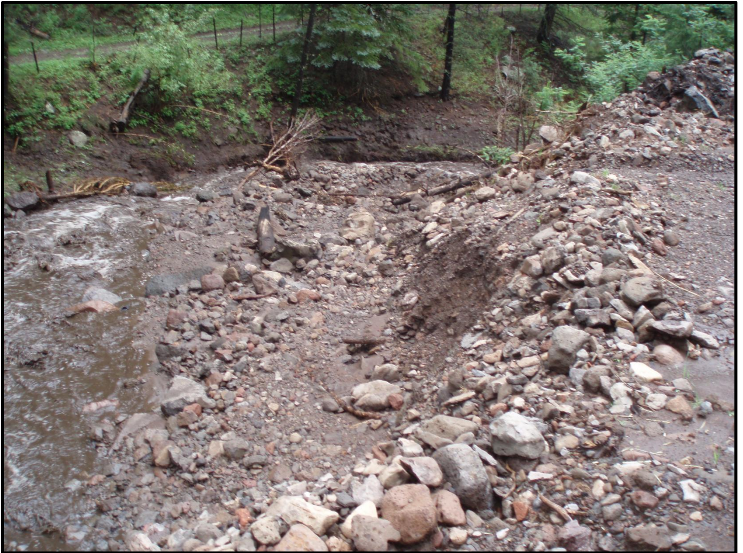
Figure 78. Looking downstream (photo provided by AZDOT, this picture was not taken on the day of the storm): This channel is below road culvert. Cross Section #3; The channel width is estimated as 20 feet wide at base, box shape with flow 6 feet deep (estimated from left bank highwater marks), wetted perimeter of 32 feet, and n value of 0.066 prior to cleaning. Slope is estimated as 0.0395 from topographic map. Estimated flow = 1,295 cfs. Mean velocity = 10.8 ft/sec.
