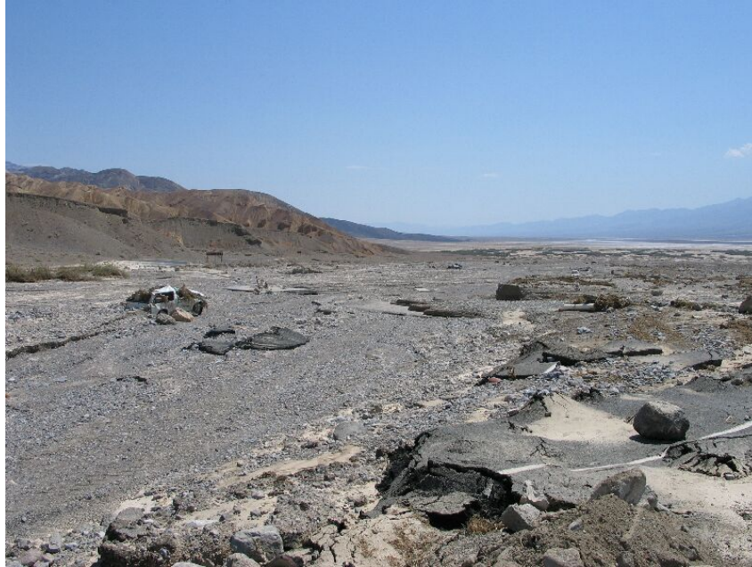
Damage at the intersection of State Routes 178 and 190. Note the extensive damage to roads and the vehicle washed away by the floodwaters. Photo Credit: Stan Czyzyk/NWS Las Vegas.
