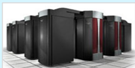
NCEP Central Operations College Park, MD (Supercomputers in Reston & Orlando)
