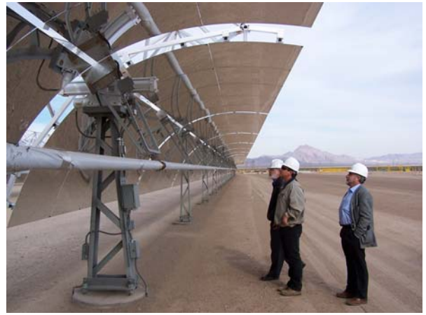
Figure 6, Nevada Solar 1 solar collector
