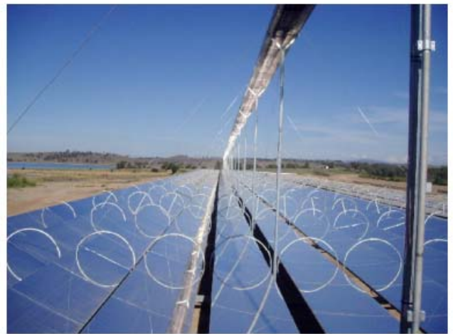
Figure 7: Linear Fresnel collector (Ausra)
