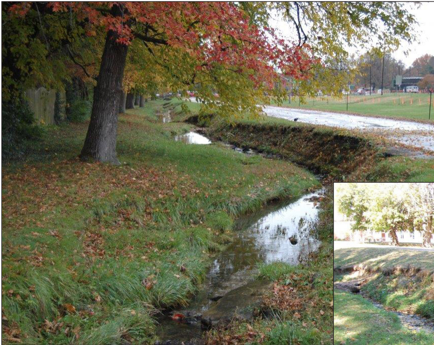
Figure 2. Eroding, unstable urban streambanks can threaten roadways and stormwater infrastructure.
