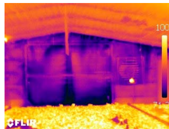
Image 1. Dark areas show air leakage at the bottom, top and center of the end door. Significant air leaks are also visible along the ceiling line at the top of the wall.
