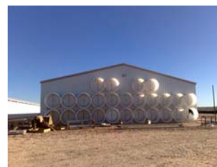
Figure 4 - Building with many tunnel ventilation fans
