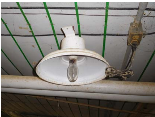
High Pressure Sodium (HPS) light
