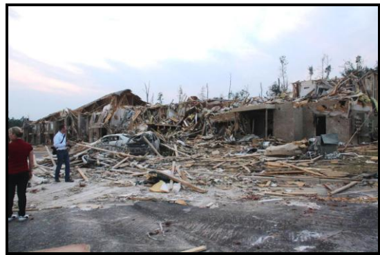
Figure 13. Ground level view looking northwest at the Chastain Manor Apartments. The tornado removed the top story.
