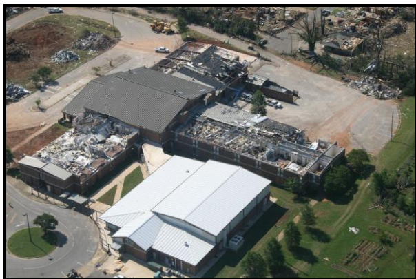
Figure 8. Aerial view of the University Place Elementary school looking southeast. Roofs over the classrooms and gymnasium were removed including many of the steel joists.
