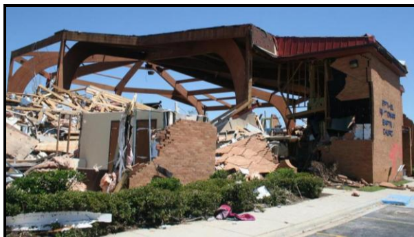
Figure 23. Tornado damage to the Bethel Baptist Church in Pratt City. The roof decking and wall framing were blown away leaving the primary glulam framing.
