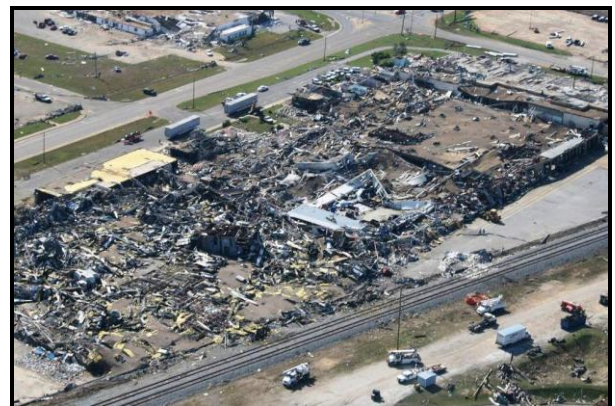
Figure 6. Collapse of the steel-framed Curry Building.
