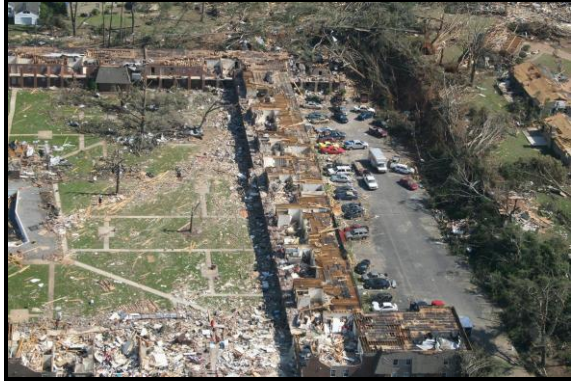
Figure 7. Removal of the roof and second story walls at the Charleston Square Apartments.
