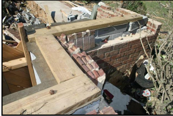
Figure 4. Sill plates were bolted to the grouted top cells in the foundation. However, the floor joists were not fastened to the sill plates.
