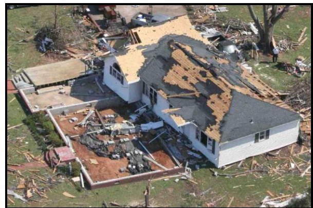
Figure 3. An unanchored home on a CMU foundation that slid into the backyard. The DOD to the roof covering suggests failure wind speeds were probably less than 45 \text{ m s}^{-1} (100 mph). Note the front porch slab remained.
