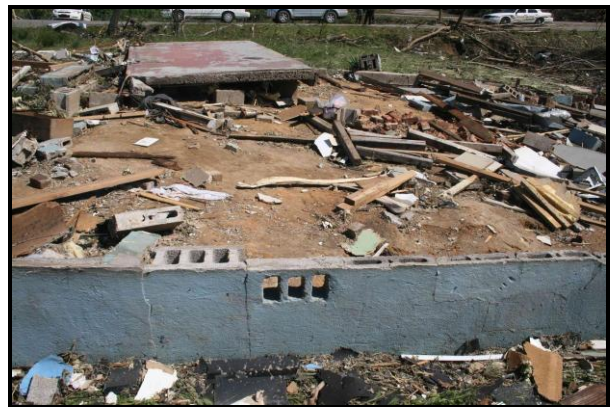
Figure 20. Unanchored home that slid off its CMU foundation. Note front porch slab remained.
