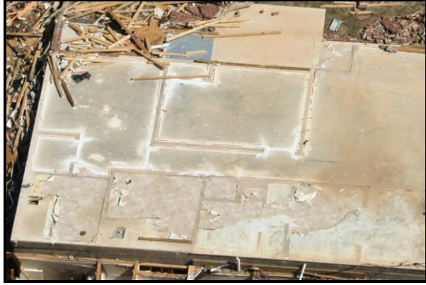
Figure 14. Closer view of the slab foundation at Chastain Manor Apartments. Wall plates were secured to the slab with cut nails instead of anchor bolts. Such connections had little pull out resistance from lateral or upward forces.
