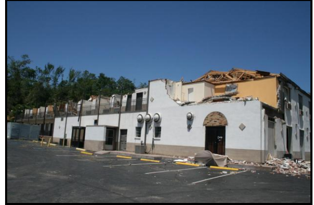
Figure 24. Tornado damage to the Super 8 Motel in Fultondale. A large portion of the roof blew away and several second story masonry walls toppled.
