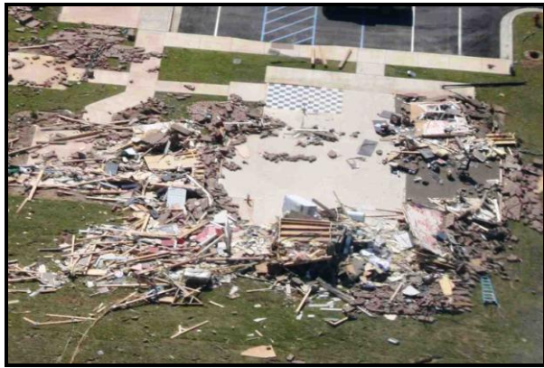
Figure 15. The office building at Chastain Manor Apartments was leveled. The walls fell outward, leaving the slab foundation exposed.
