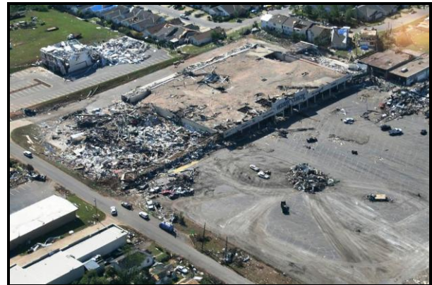
Figure 9. Northwest elevation view of the Wood Square Shopping Center. Large portions of the building collapsed.
