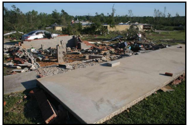
Figure 19. An unanchored home on a CMU foundation. The front porch slab (foreground) and vehicle (background) remained although the unanchored slab did shift.
