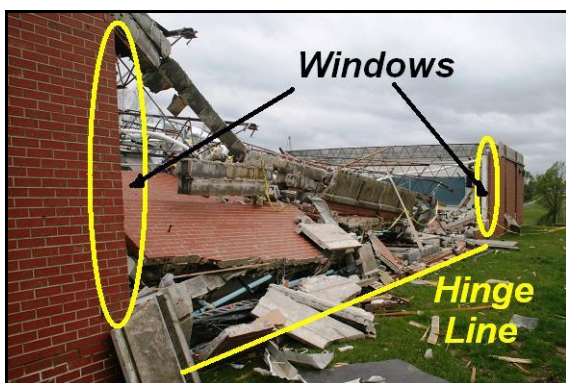
Figure 17. Collapsed north wall on the west wing of the high school. The wall collapsed about a hinge line at the base of the wall. Tall window openings (circled) created weak vertical joints in the wall.
