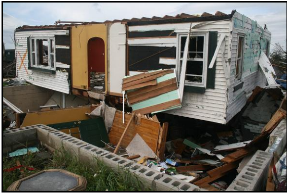
Figure 13. Unanchored home that slid off its CMU foundation was rated EF-2 due to loss of its roof.
