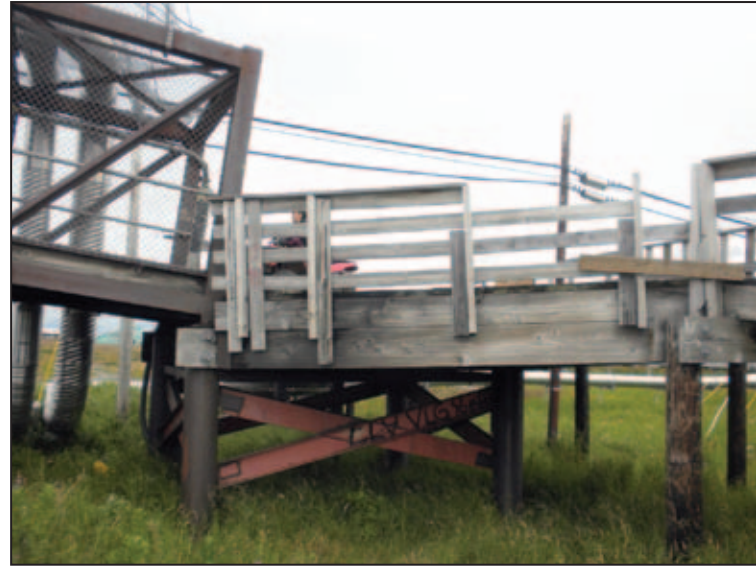
Evidence of movement on Rainbow Bridge ramp. Mike Brubaker, 2011.
