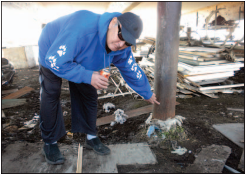
Lawrence Larkin point to original ground level under his home. Mike Brubaker, 2011.
