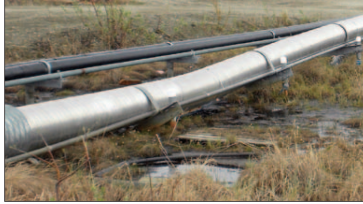
Arctic pipes, sagging as they sink into the ground. Mike Brubaker, 2011.
