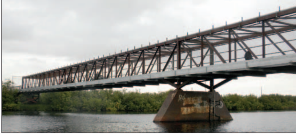
Rainbow bridge is one of two large bridges that are thought to be sinking. Mike Brubaker, 2011.
