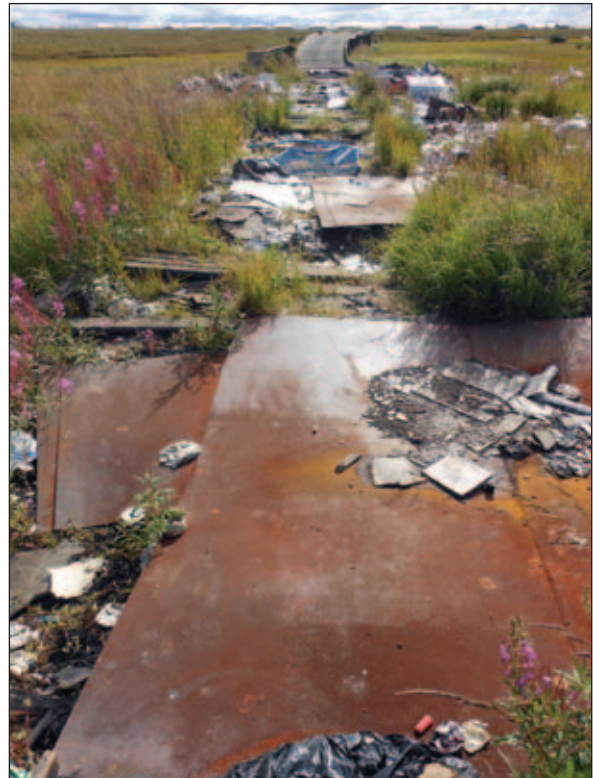
A damage section of the dump board road. Raj Chavan, 2011.
