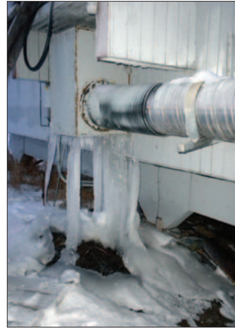
Broken water pipes. Mike Brubaker, 2011.
