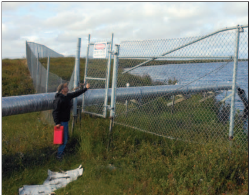
Sinking and erosion has damaged the sewage pond outfall. Raj Chavan, 2011.
