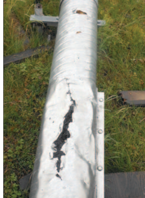
A vehicle damaged Arctic pipe. Mike Brubaker, 2011.
