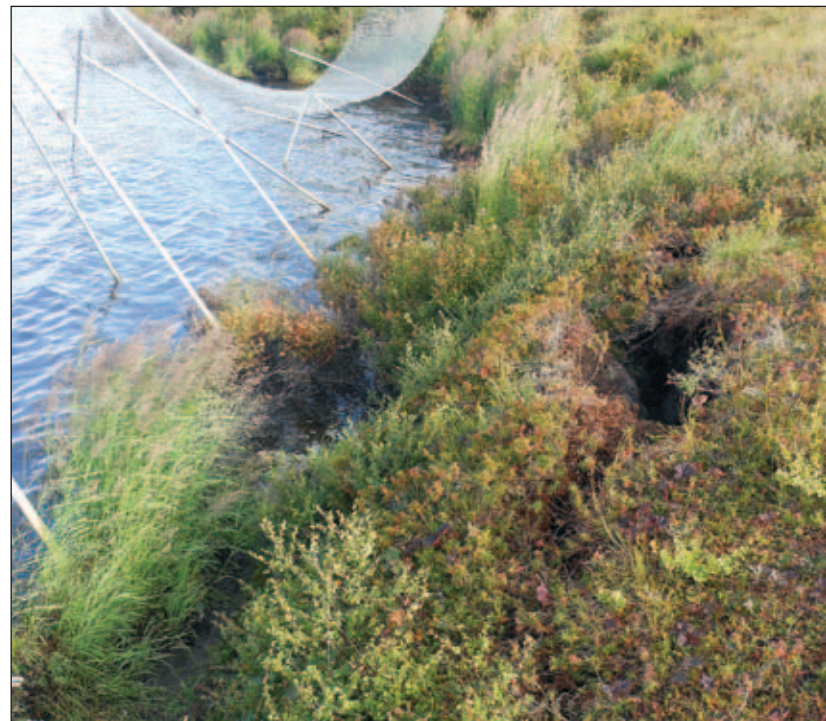
Erosion at the sewage pond. Raj Chavan, 2011.
