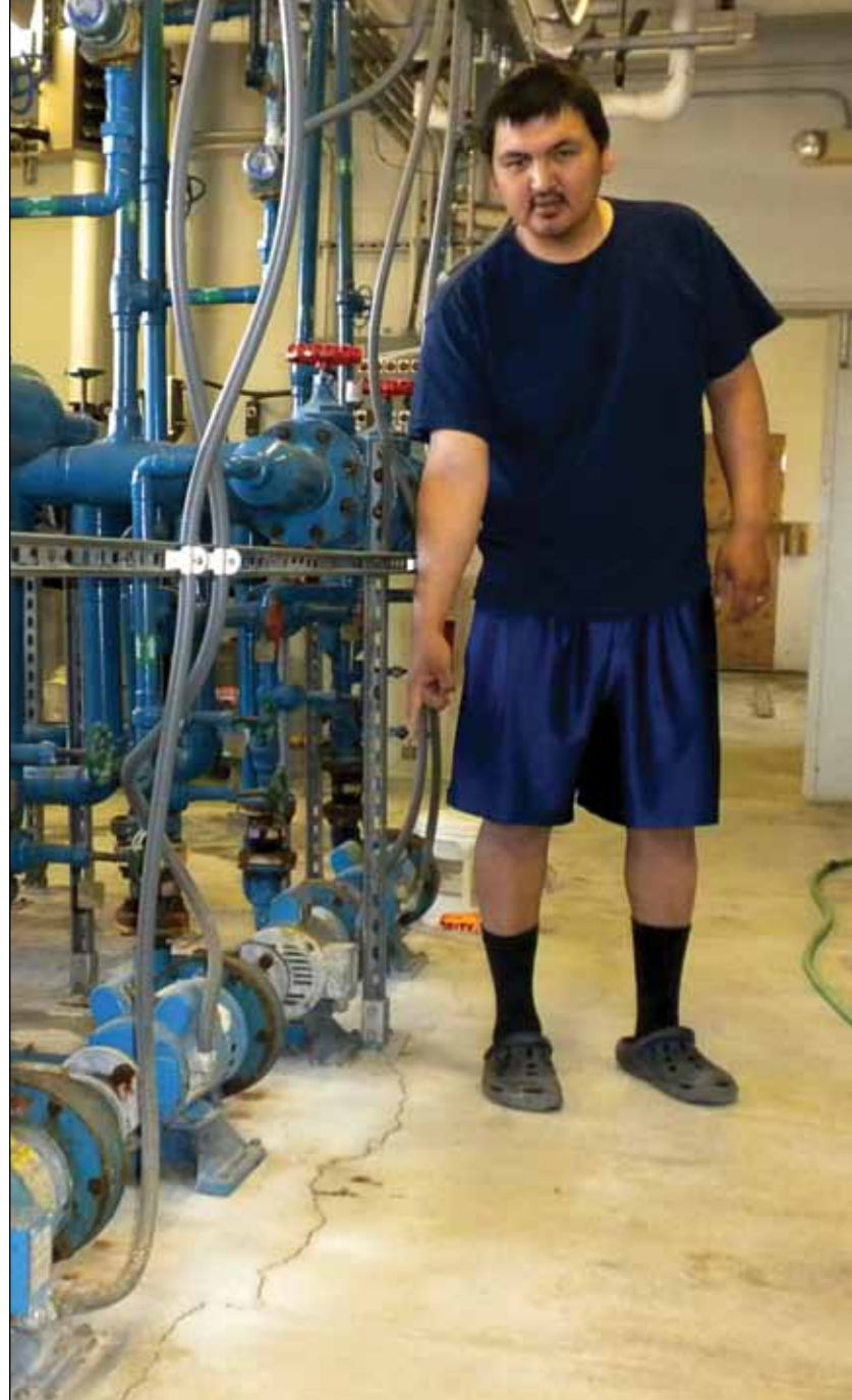
Jeffery Luther shows foundation crack in water plant. Ryan Brubaker, 2010.
