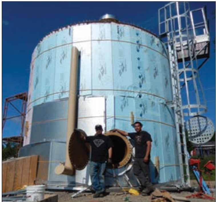
New water storage tank under construction in Nondalton. Photo by Mike Brubaker, 2013.
