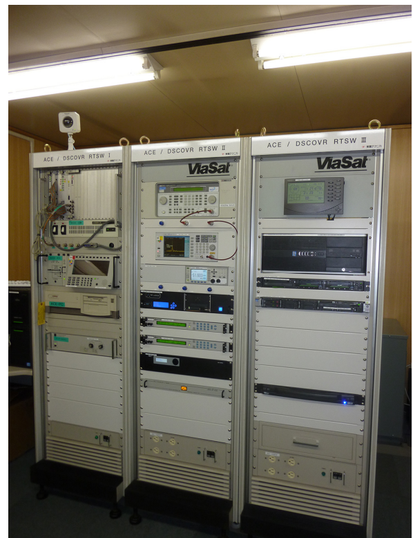
The Antenna control and data receiving system
