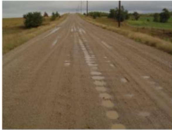
Figure 3.21 Gravel road with inadequate crown
