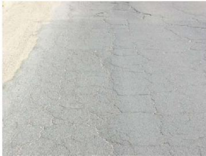
Figure 3.9 Example of alligator cracking, moderate severity.
