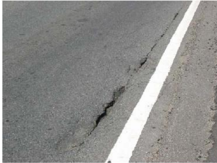
Figure 3.7 Example of longitudinal and transverse cracking, heavy severity
