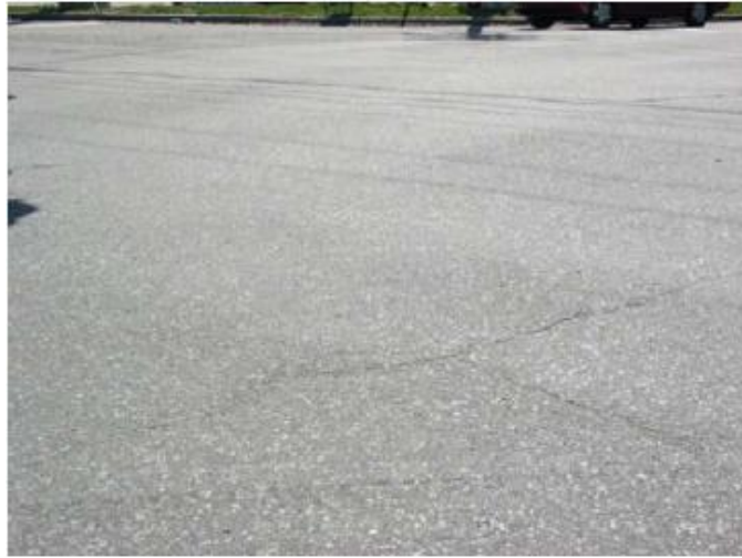
Figure 3.5 Example of longitudinal and transverse cracking, slight severity.
