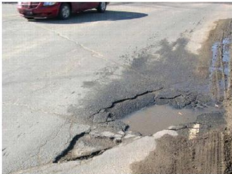
Figure 3.16 Example of potholes, high severity
