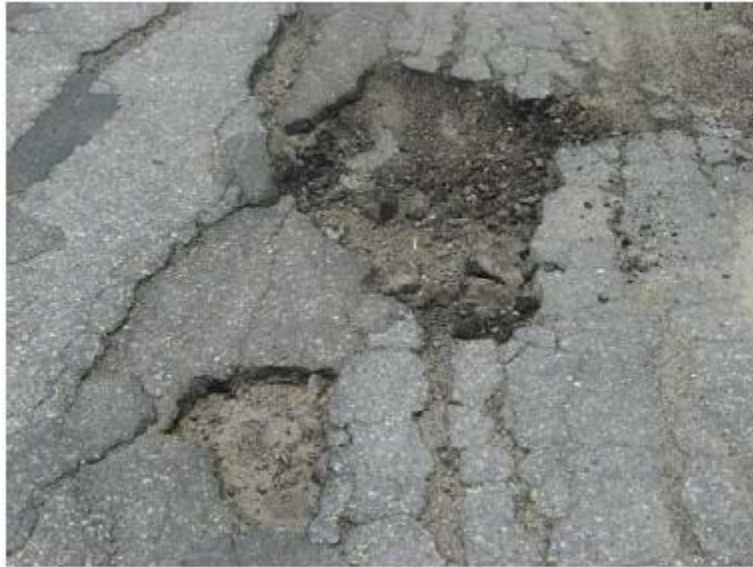
Figure 3.15 Example of potholes, moderate severity
