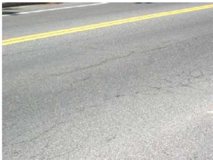
Figure 3.8 Example of alligator cracking, slight severity
