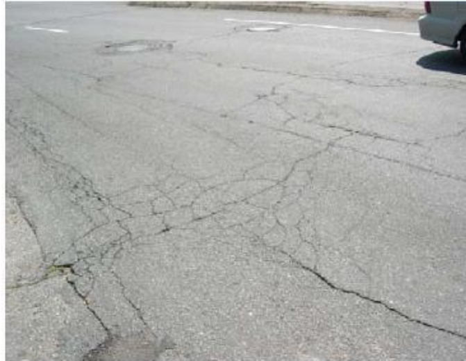
Figure 3.13 Example of block cracking, high severity.
