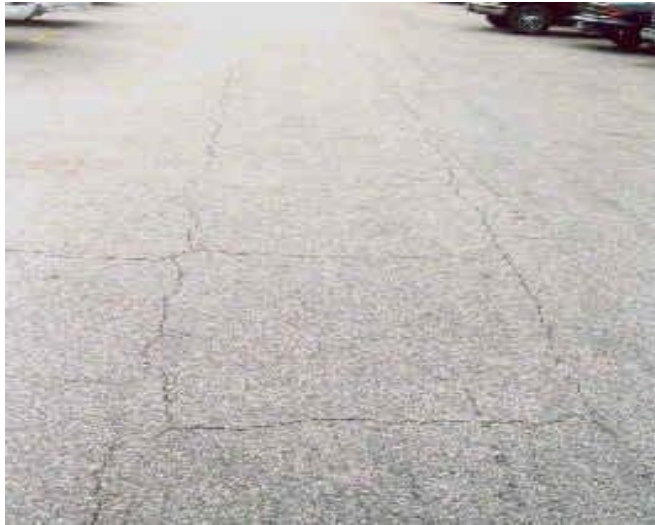
Figure 3.11 Example of block cracking, slight severity.
