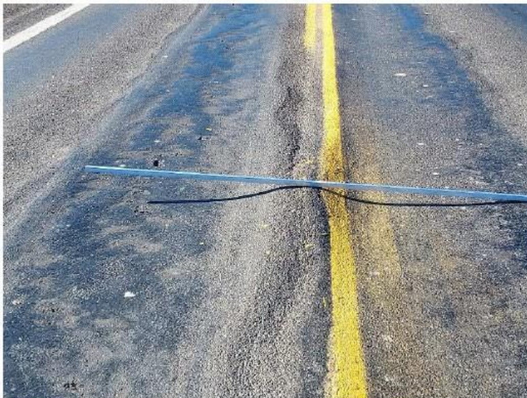
Pavement conditions in rural Idaho. 3700 North near Twin Falls, ID.
