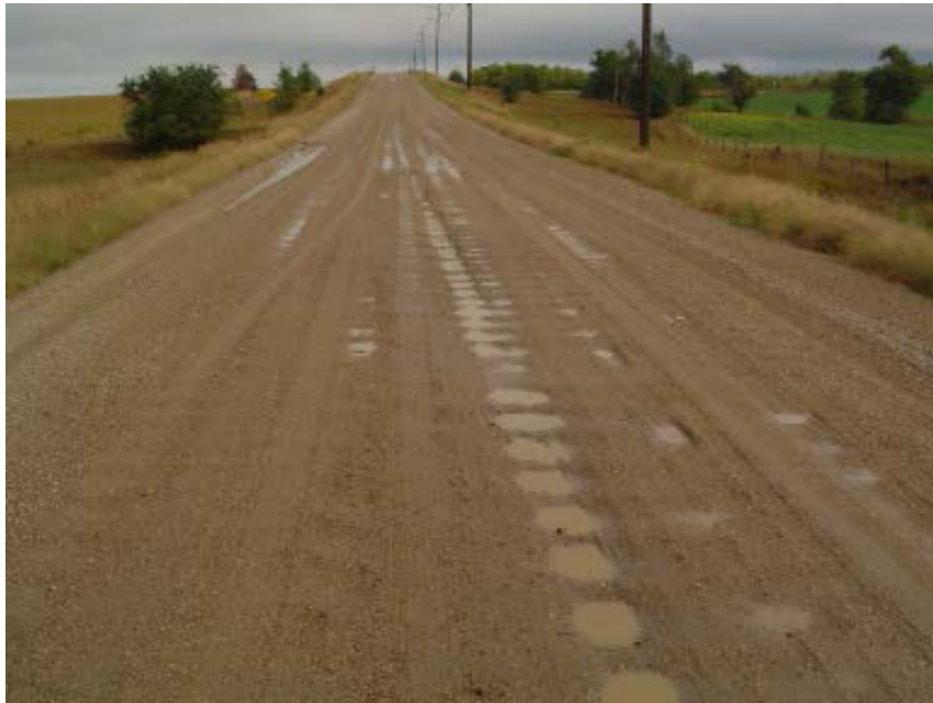
Figure 9: Gravel road with inadequate crown.
