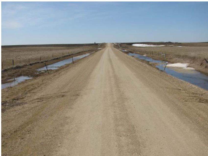
Figure 10: Gravel road with excessive crown.
