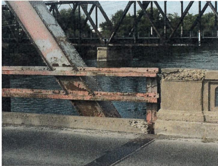
Figure 4. Deteriorated Concrete and Paint
