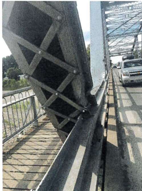
Figure 3. Example Girder Damage
