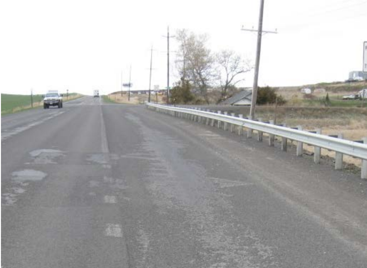
Snowplow: CODs Exacerbated by Snowplows – Unacceptable
