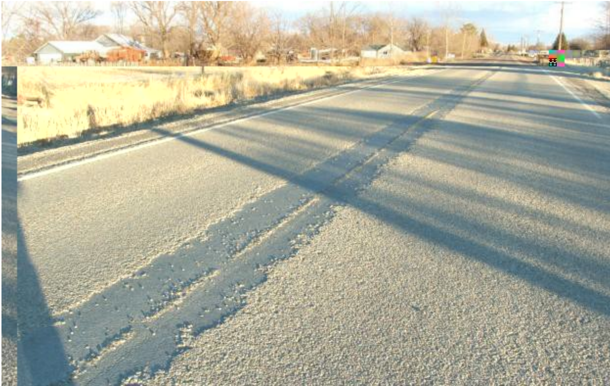
Longitudinal Joint: Unacceptable chip loss (CODs)
