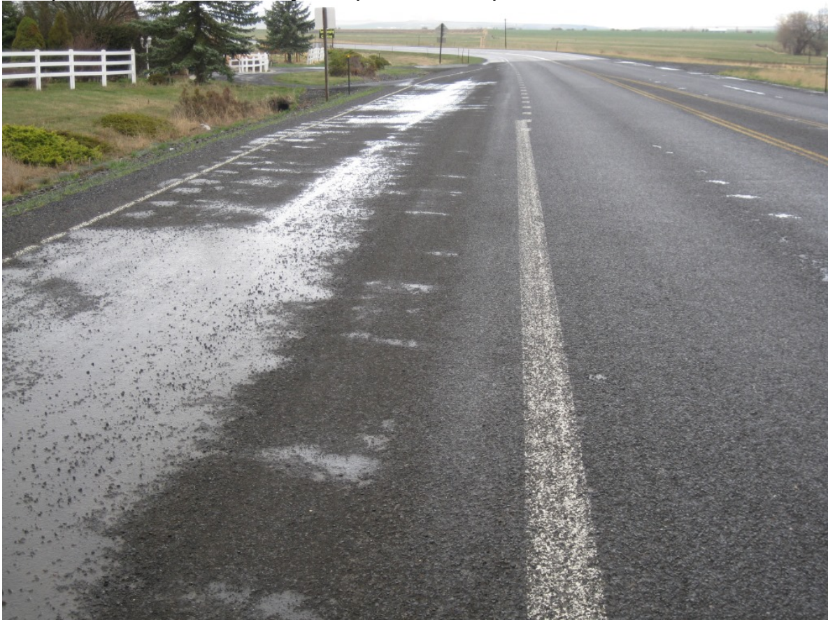
Snowplow: CODs Exacerbated by Snowplows – Unacceptable
