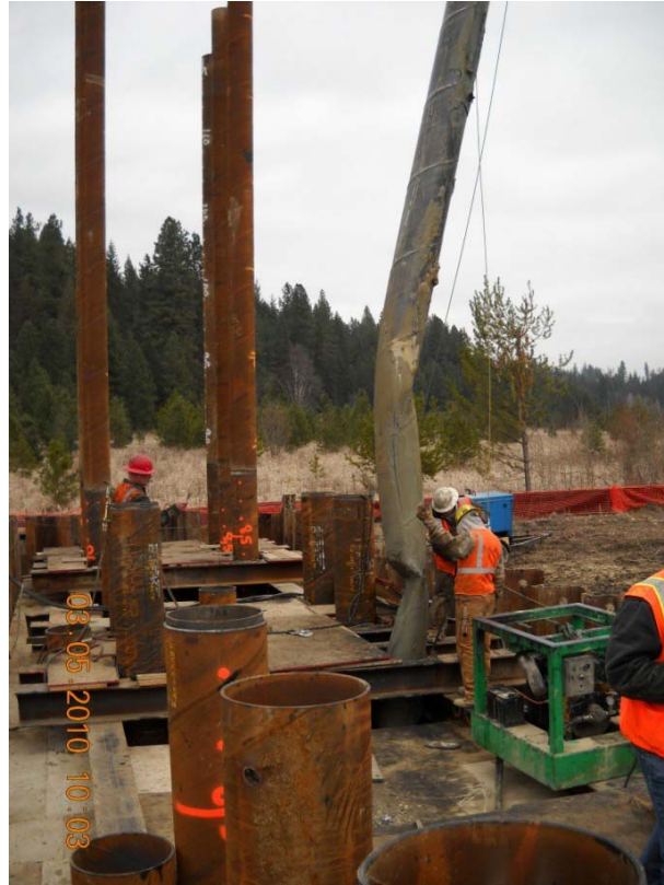
Photo 4. Pipe pile damaged on sloping rock surface, in the process of being extracted.
