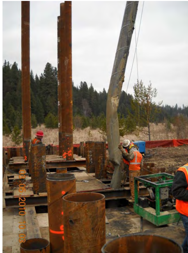
Photo 4. Pipe pile damaged on sloping rock surface, in the process of being extracted.
