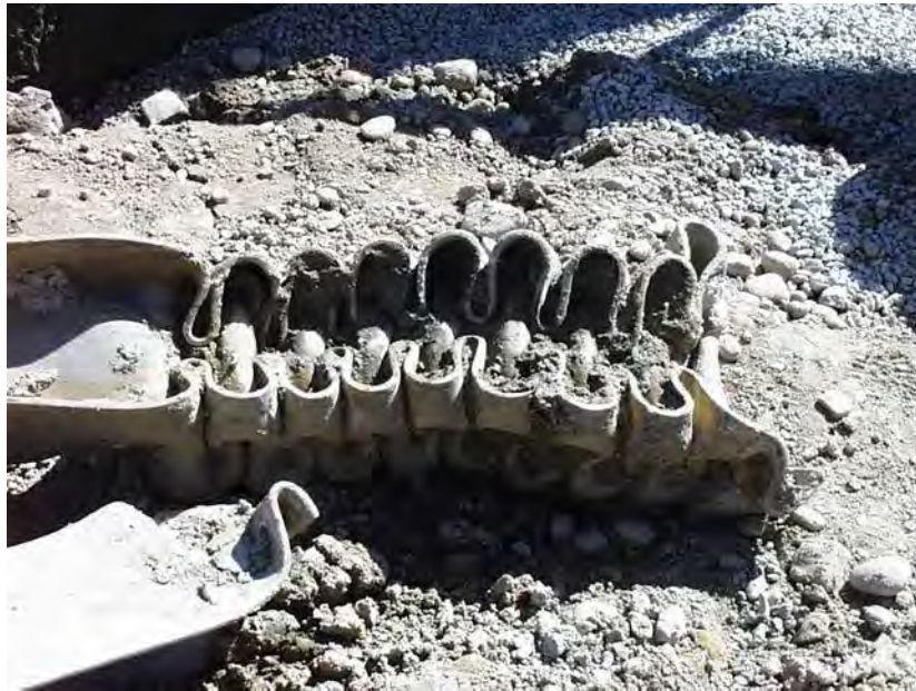
Photo 3. Damaged H pile due to overdriving.
