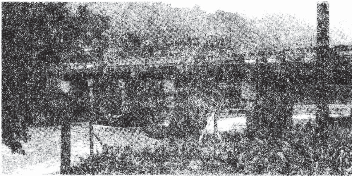
Bridge in Hazard, Kentucky With Multiple Piers Inoperable as the Accumulation of Flood Debris.
