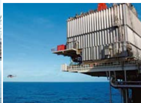
HVDC Light Module on Troll-A platform (ABB)
