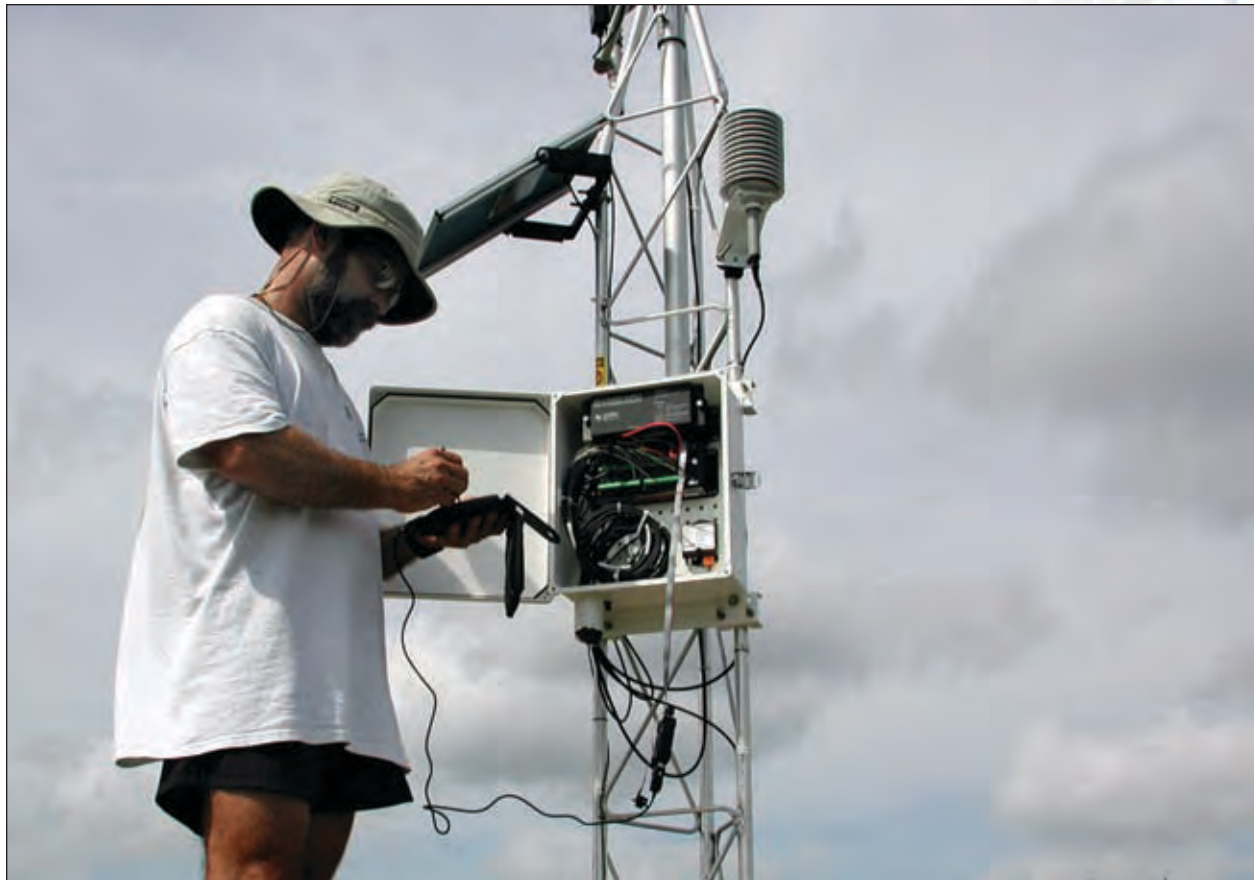
Real-time monitoring of weather conditions contribute to a nationwide network of climate change information being compiled by the National Estuarine Research Reserve Program.
