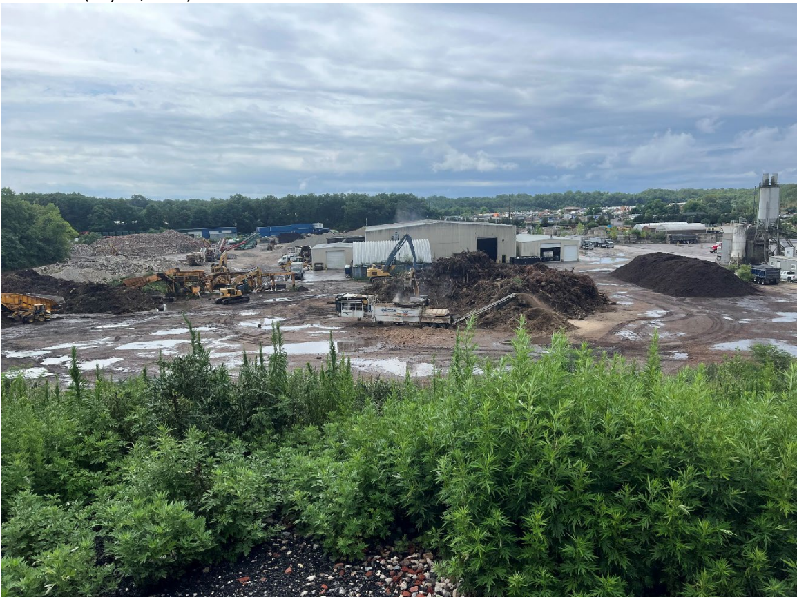
Photograph No. 2: View of site operations at the Project Area, facing south (July 14, 2023).
