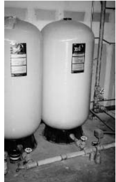
Figure 5.7 Captive air tanks
