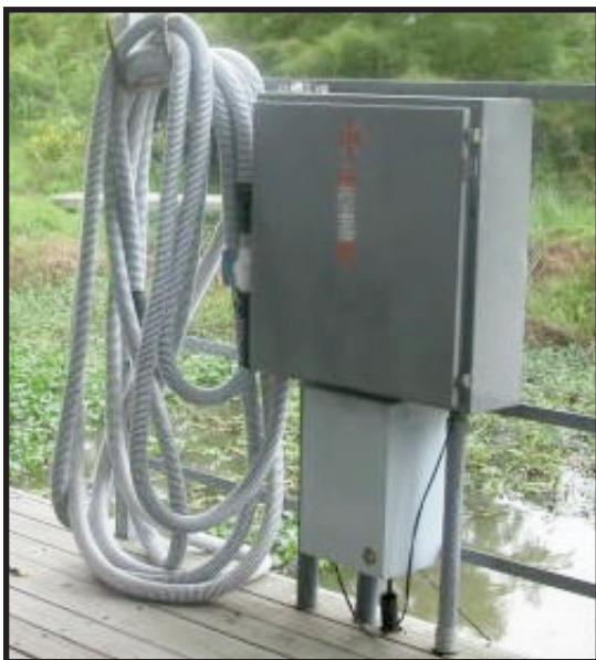
A stand-alone unit is hooked up to the hydrant at a dock using a slip-to-slip pump-out.
