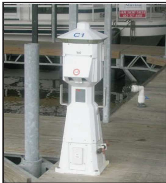
A stand-alone slip-to-slip pump-out unit located in the middle of the dock provides the boater with a convenient method of pumping out.
