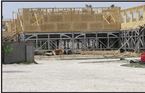
The Grand Bay NERR is constructing a new $7 million reserve facility, the Grand Bay Coastal Resources Center.
