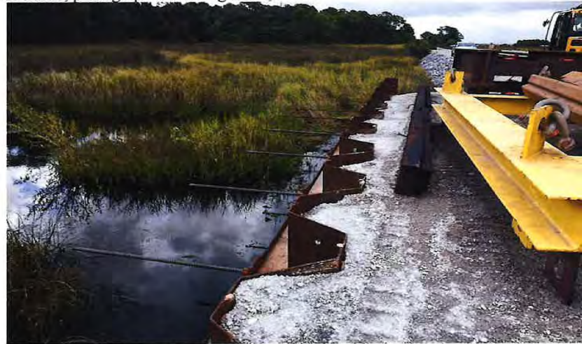
Photograph 4: view of recently backfilled LTP; note access route in background; facing west from north side of tracks; photograph taken August 30, 2018.
