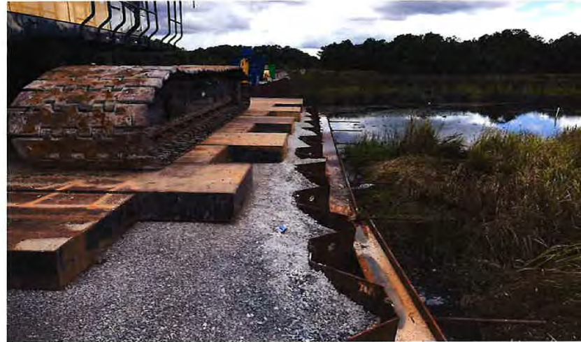
Photograph 3: view of recently backfilled LTP with crawler crane in-place; note additional steel crane mats required to distribute loading; facing east from north side of tracks; photograph taken August 30, 2018.
