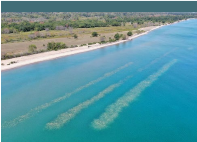
Aerial view of fully installed submerged rubble ridges at Illinois Beach State Park. Photo credit: US Army Corps of Engineers
