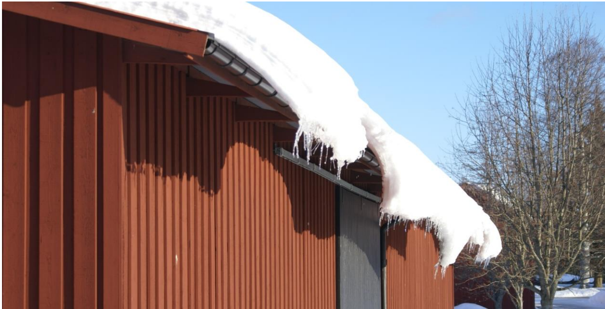
Figure 48: Picture taken on heavy snow and ice formation in spring in BJURÅS, Northern Sweden. Later, the frame showed a damage as in Figure 49 [Courtesy of Klaus Lorenz Högskolan Dalarna].
