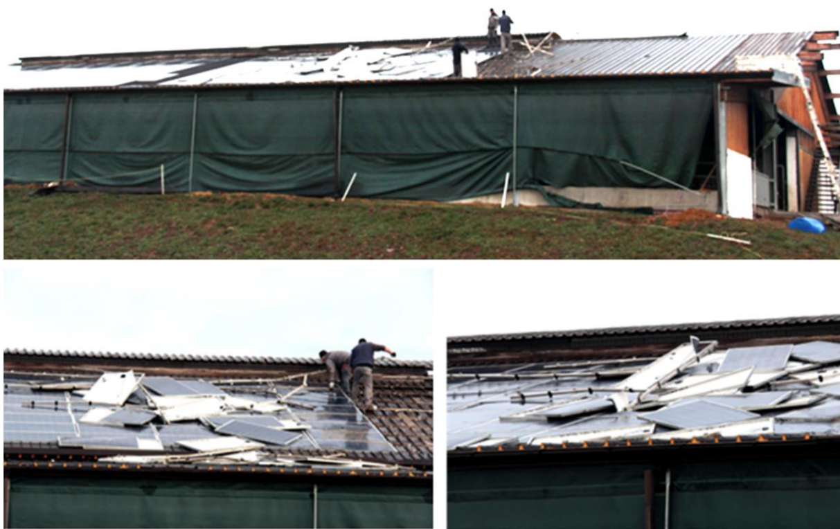
Figure 44: PV System status after a windstorm in Baselga di Piné, Italy. Source: Dino Loriatti.
