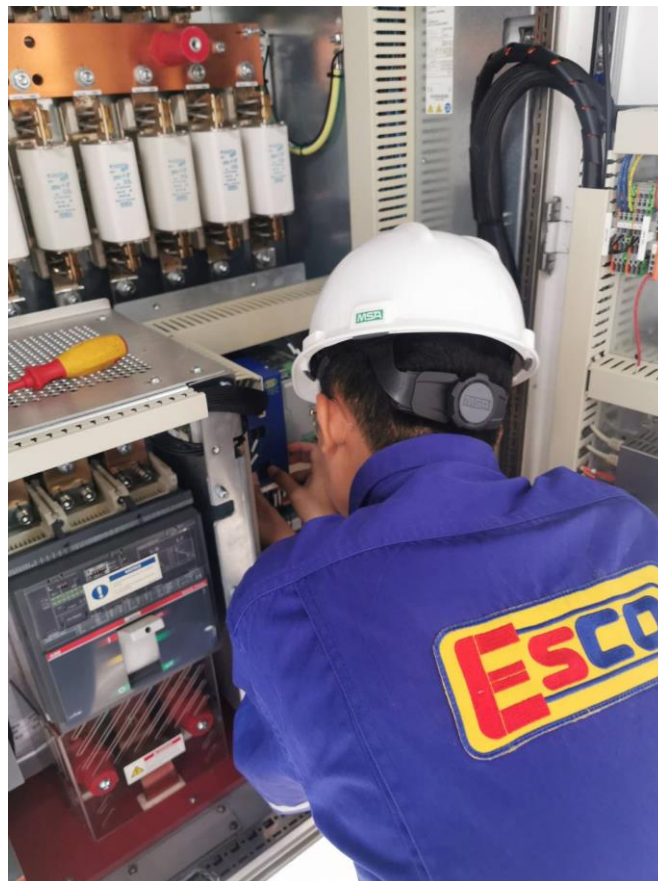
Figure 32: Regular checking and performing preventive maintenance in PV power plants in Thailand.
