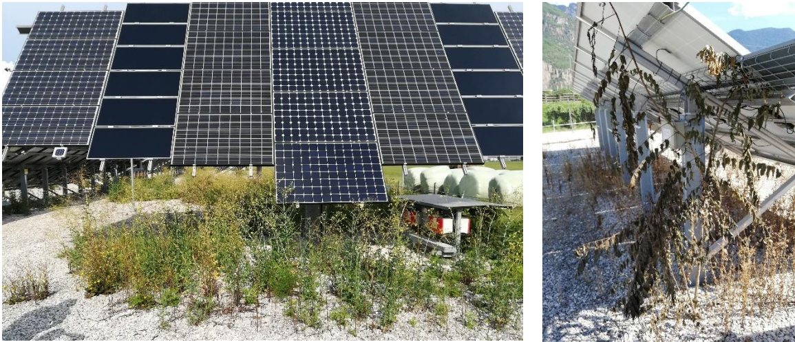
Figure 11: Growing bush in front of a tracker (left) and underneath an array (right) [Eurac Research].
