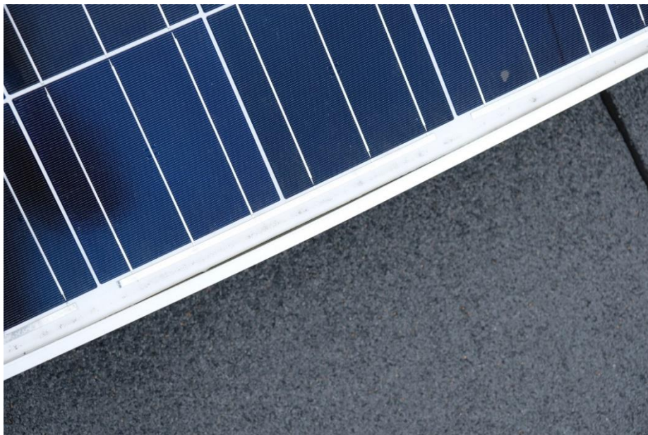
Figure 49: After winter, loose frames were observed on PV modules in Piteå in Northern Sweden [Picture from Mats Axelsson].
