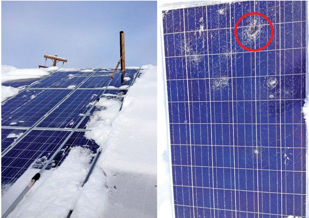
Figure 52: Careless removal of snow may destroy the surface of PV modules [166].
