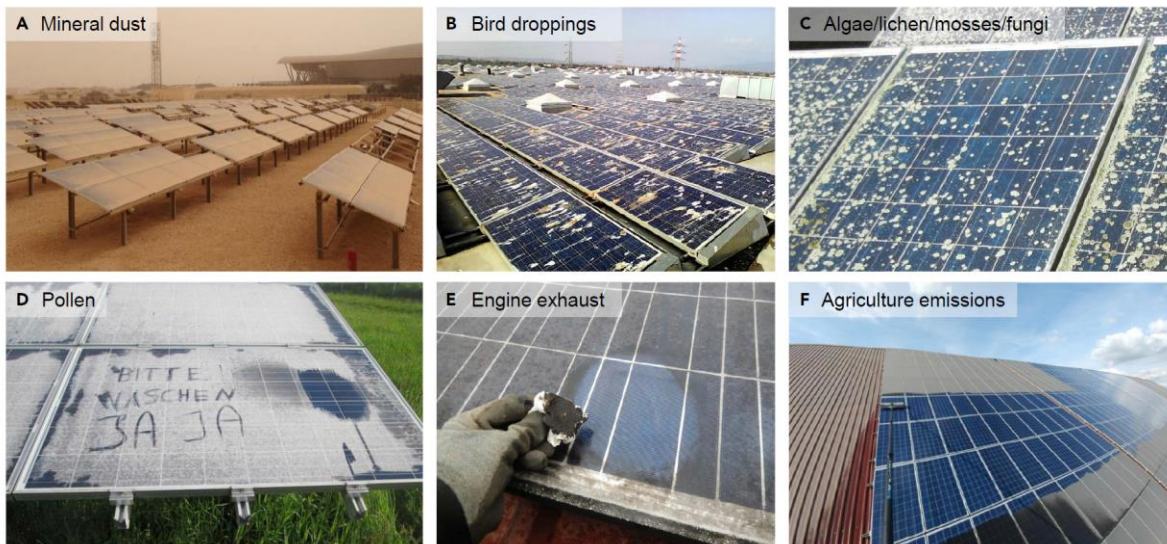
Figure 13: Examples of different types of soiling of PV arrays [83].
