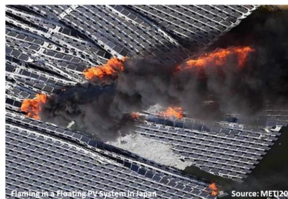
Figure 42: Damages of PV facilities by typhoons in Japan in 2018 and 2019.
