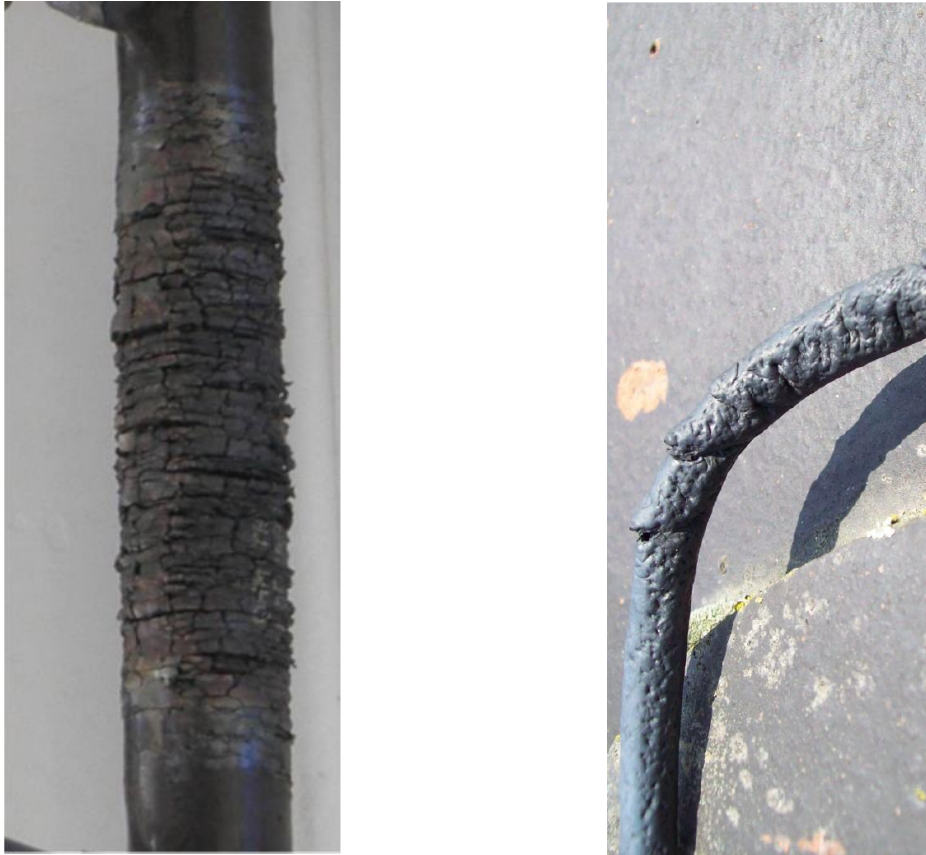
Figure 26: Examples of damages in cables in power plants located in the Atacama Desert.
