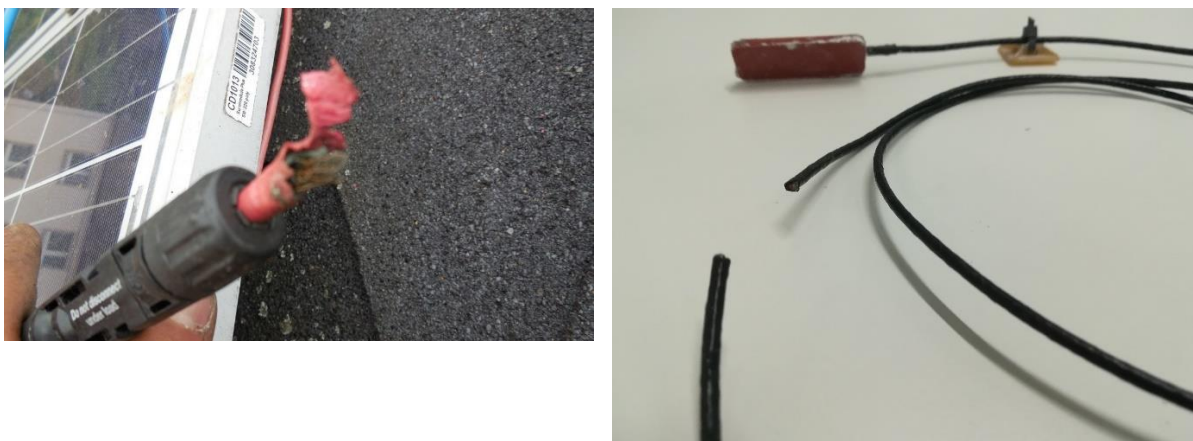
Figure 12: Cable bitten by a marten (left) (pveurope.eu © Leitl). Temperature sensor cable cut in half by a rodent (right) [Eurac Research].
