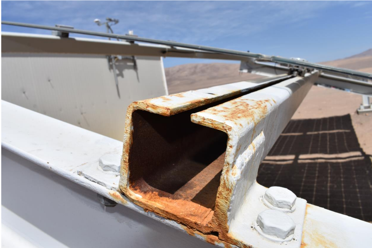
Figure 28: Rusted mounting structure in a PV power plant located in the Atacama Desert. This mounting structure has been in operation for about one year.
