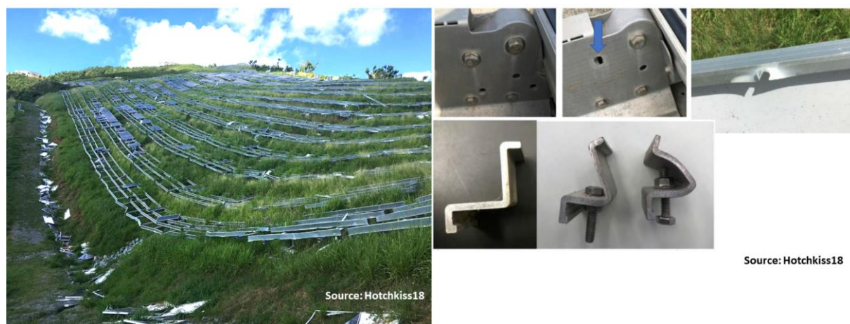
Figure 43: Damages of PV facilities by hurricanes in U.S. Virgin Islands in 2017.
