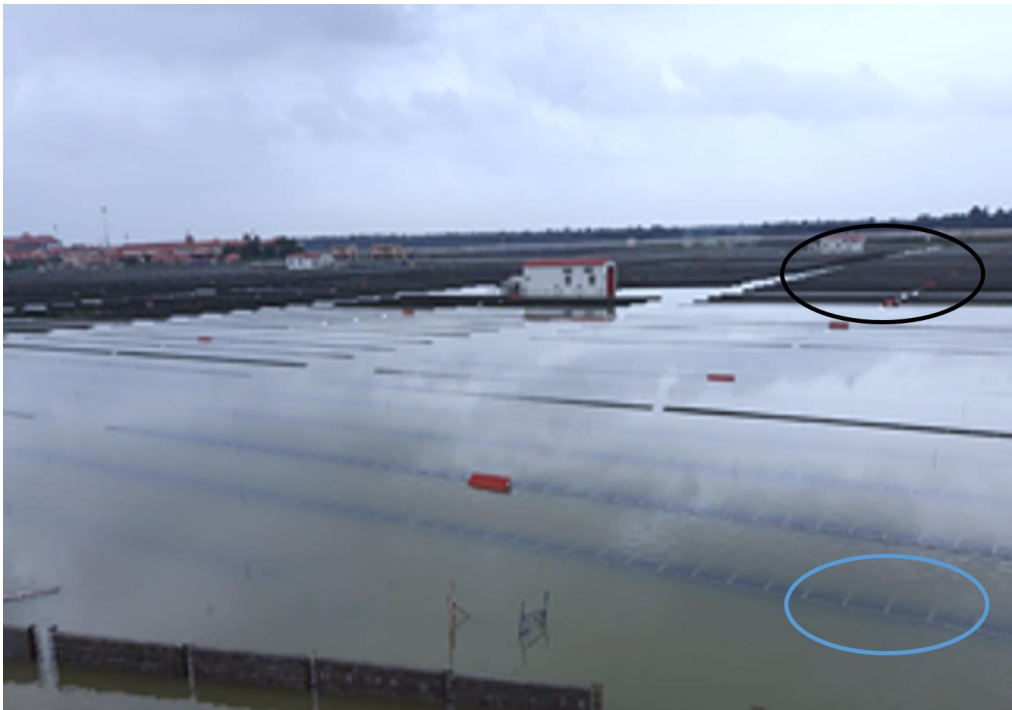
Figure 33: Partially submerged PV plant showing strings fully submerged in water (in blue circle) and those that are above water (in black circle).
