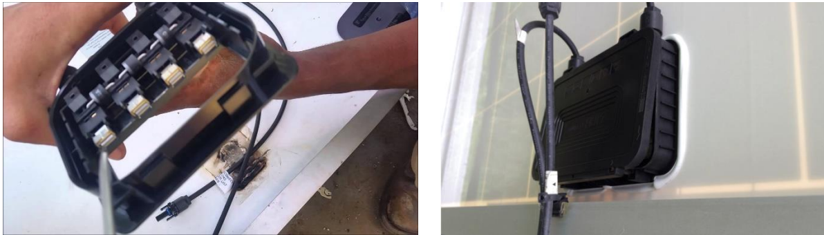
Figure 27: Failures in a junction box in operation during about a year due to degradation issues.
