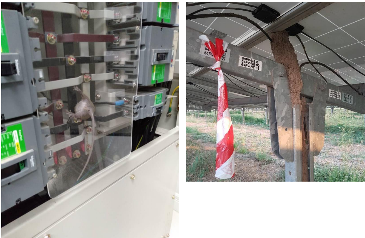
Figure 30: Impact by wildlife on PV components, such as a rat in the main distribution box (left) and termites around the DC cable under the PV module (right).
