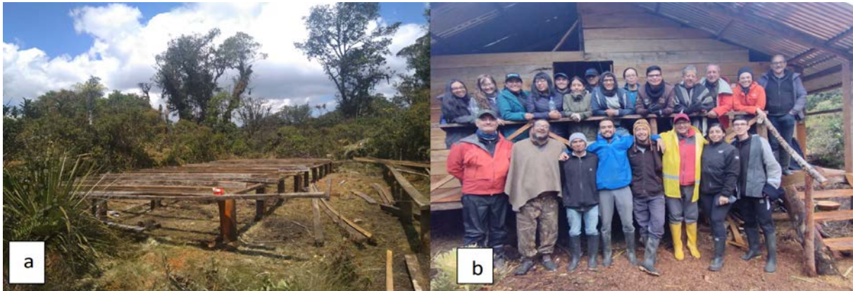
(a) basement of the building and (b) finished meeting room with participants of the workshop
