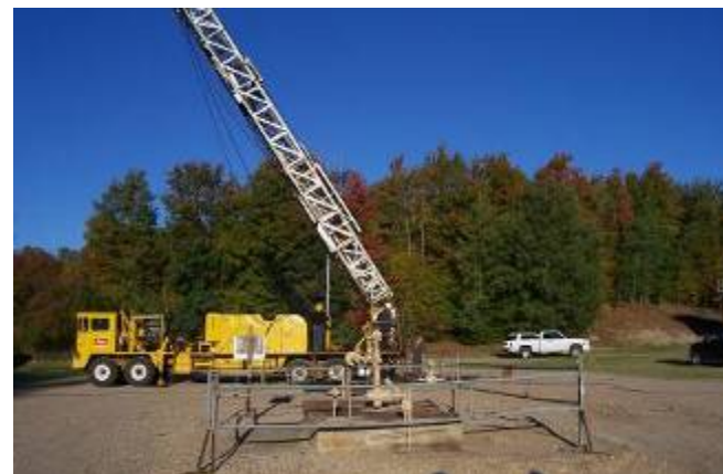
Monitoring Well (about 500 feet from injection well)
