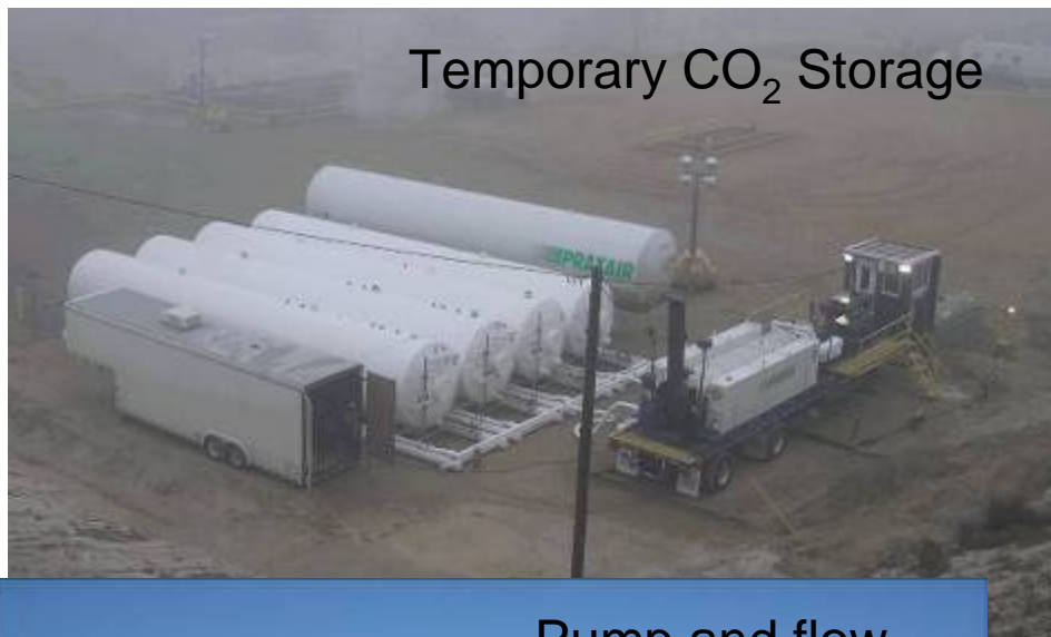
Pump and flow control equipment
