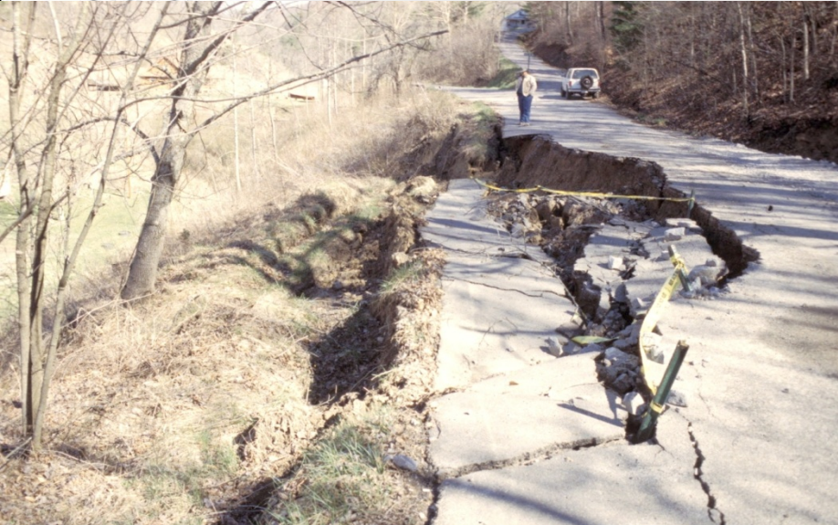
Road Failures on Shale
