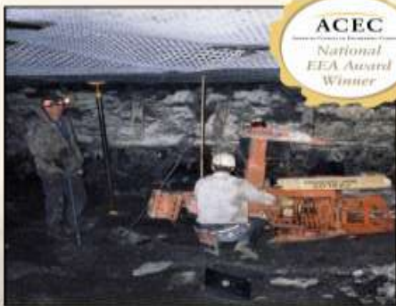
Installation of high-strength fiber mesh/resin roof bolting system for stability and safety
