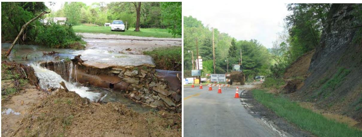
Figure 3.49. Examples of large wash outs of sediment during heavy rain events. The photo on the left is private drive that crossed a minor tributary of Christy Creek near CC-2.00. The photo on the right is a hillside on HWY 32 near the bridge that crossed Triplett Creek.
