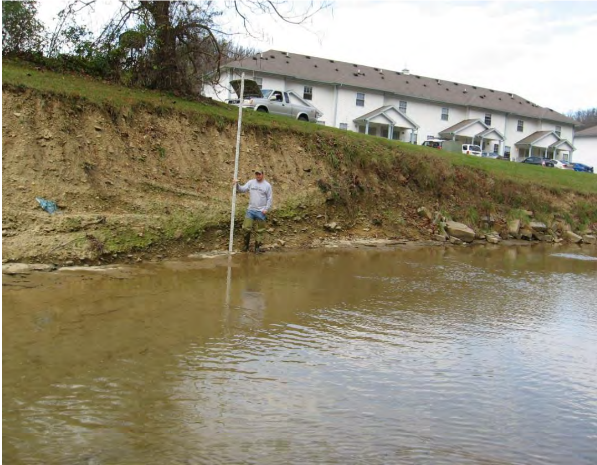
Figure 3.53. Example of a streambank with extreme erosion risk (MBEHI = 35.0).
