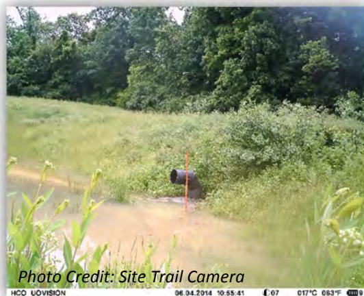
Figure 4-5: Detention basin retrofit at Toyota site during storm event on June 4, 2014.
