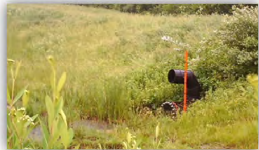
Figure 5-10: Detention basin retrofit technology cost-effectively optimizes excess capacity for downstream channel stability
