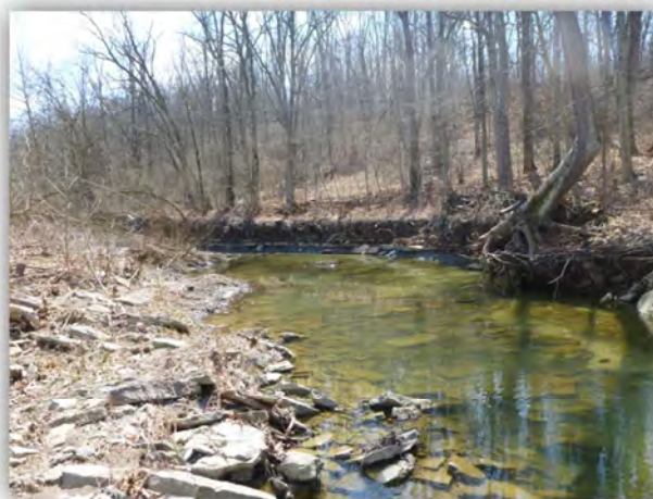
Figure 1-1: The impacts of hydromodification in the Allen Fork Subwatershed are illustrated by the eroding streambank
