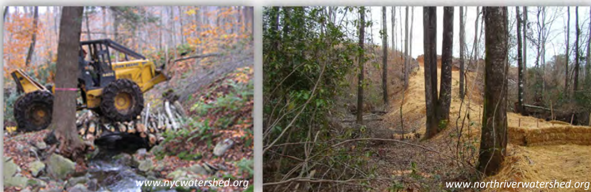
Figure 5-4: Forestry BMPs: Use of a culvert for stream crossing (left) and erosion protection using straw and bales (right)
