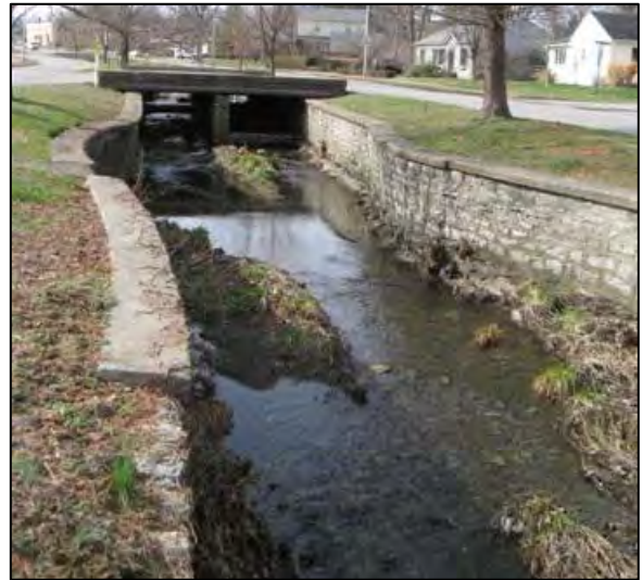
Armored Banks on Wolf Run at Lafayette Parkway
