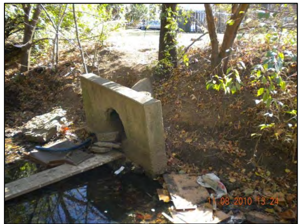
Erosion and Infrastructure Damage at Vaughn's Branch Mouth
