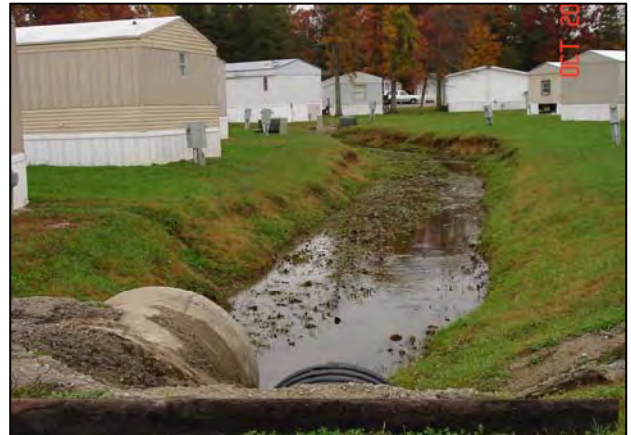
Channelized Section of Sampson Branch (Little Laurel Subwatershed) with Indications of Bank Erosion
