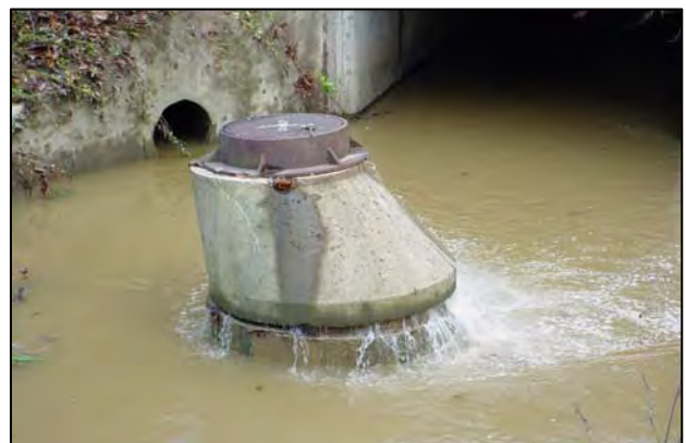
Sanitary Sewer Overflow on Whitley Branch
