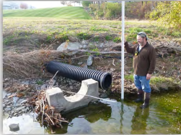
Figure 4-11: Storm sewer infrastructure at Site SFG 5.3-DS compromised by erosive, urban flow regime
