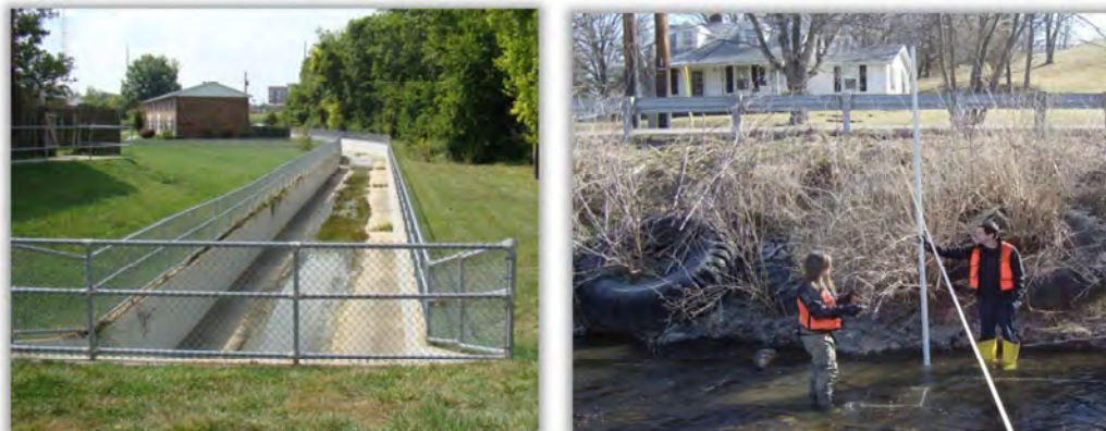
Figure 2-8: Artificial channel armoring such as concrete (Utterback Creek off Industrial Road) and tractor tires (South Fork of Gunpowder along Gunpowder Road near Sunnybrook Drive) reduce habitat quality and stream integrity
