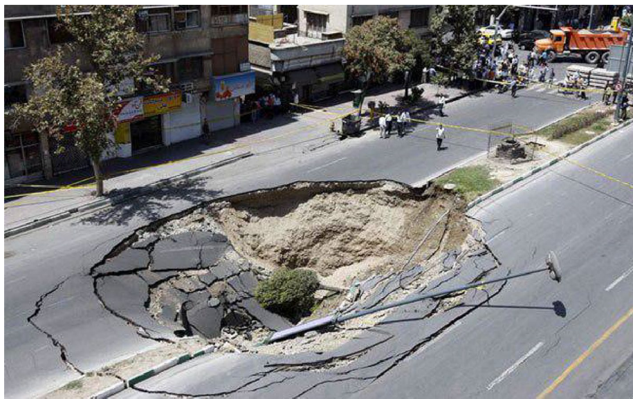
Fig. 21 Collapsed aqueduct near Navab Square, Tehran (east of HSHT)
