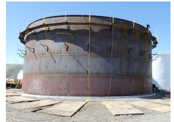
Storage tank at incident site.
