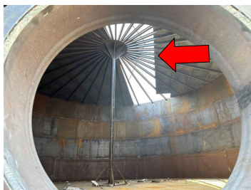
Hole in roof where welder fell.
