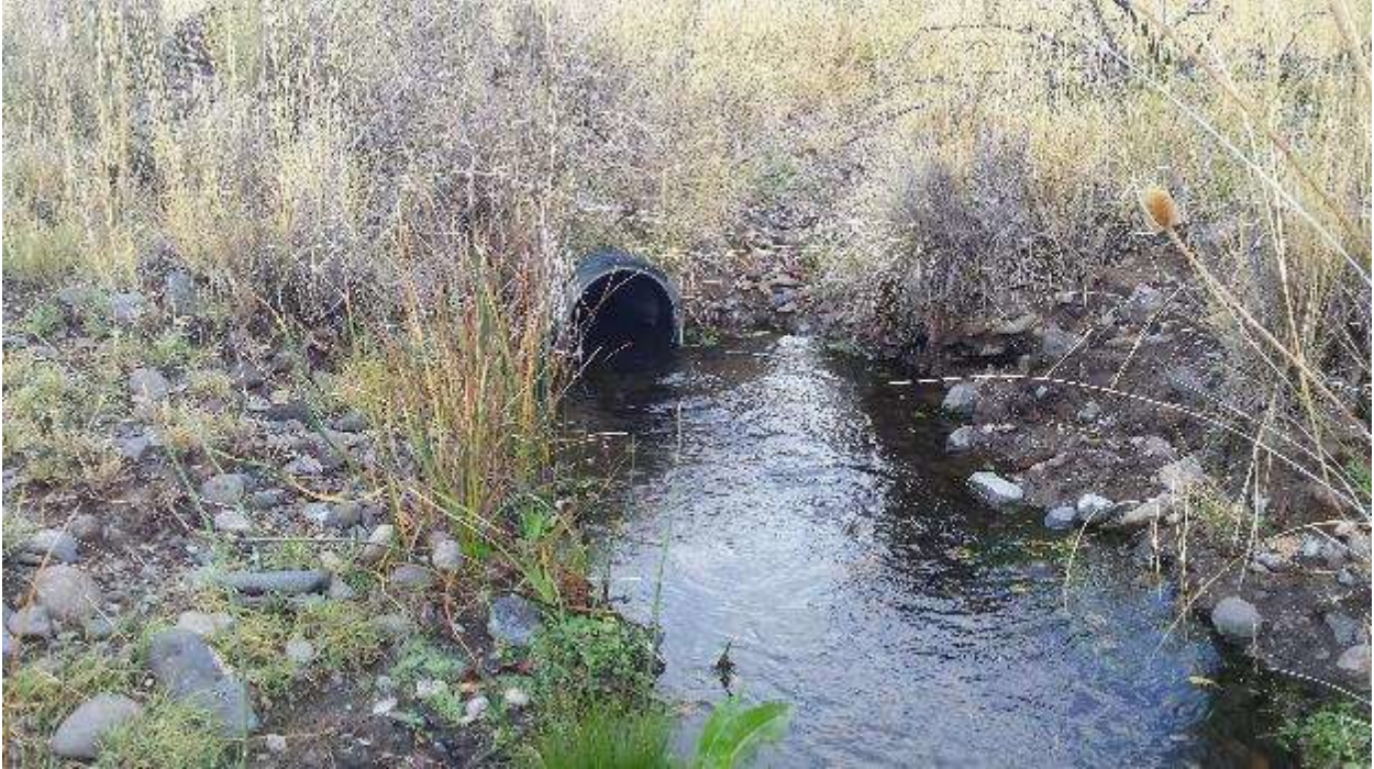
Photo 7 – Fish Return Pipe at Musgrave Diversion.
