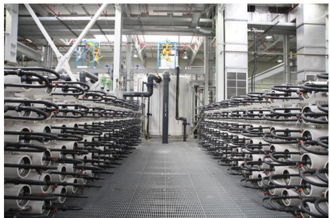
Figure 2 GWRS reverse osmosis trains (Photo Credit: Gina DePinto)
