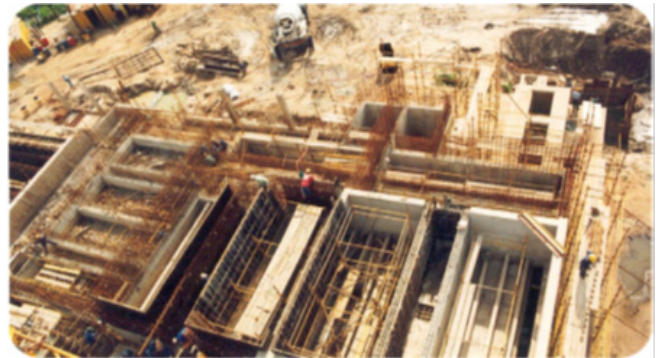
Figure 1 Construction of the Durban Wastewater Recycling Plant (Photo credit: Ethekeeni Metro Water Services)
