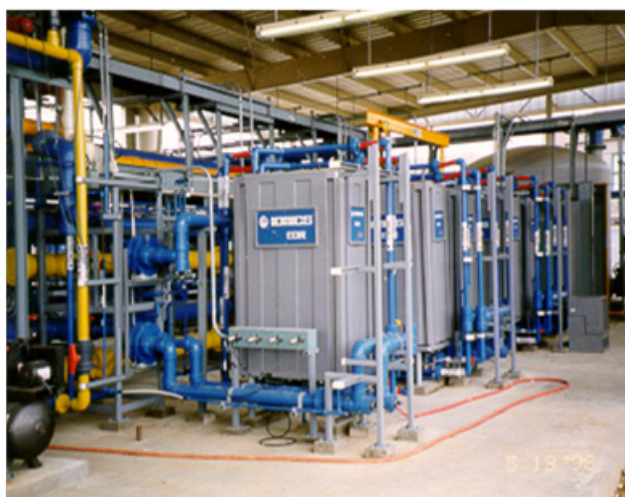
Figure 1 North City WRP with 6th EDR unit installed
