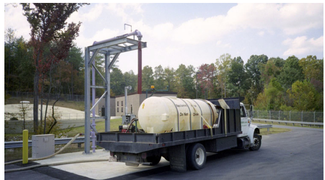
Figure 1 Bulk reclaimed water distribution station (Photo credit: David Heiser)
