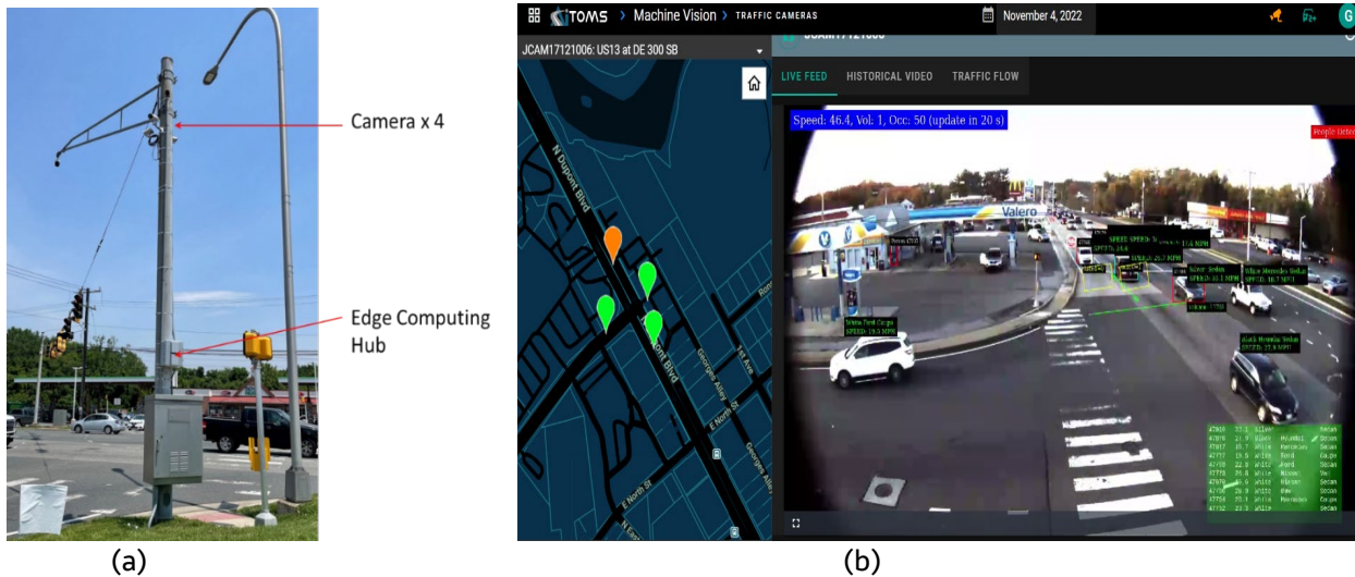
Figure 5. (a) BlueHalo’s Edge Computing multi-channel machine vision cameras installed at US-13 @ DE-300 in Smyrna, DE; (b) the web portal for the machine vision cameras for vehicle count, classification, and speed and occupancy estimation
