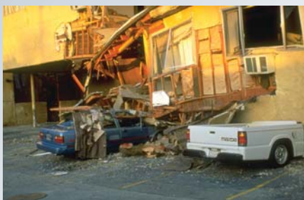
The first story of this apartment building collapsed, crushing cars below (FEMA photo).
