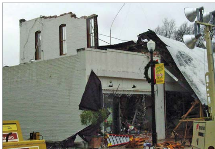
Collapsed roof in downtown Paso Robles following the San Simeon earthquake of December 22, 2003. Two people were killed by falling debris when they ran out of the building. (USGS photo)
