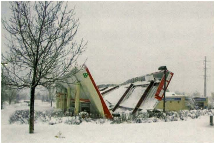
Gas Station Canopy Collapse. Photo by G. Merlo.
