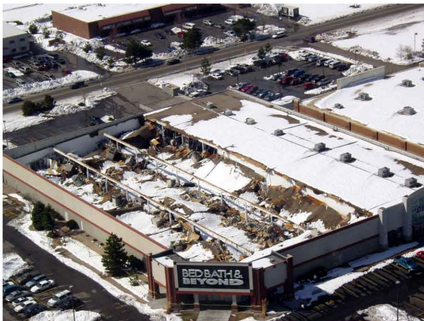
Figure 11. Collapsed roof of the large Bed, Bath, and Beyond store on south College Avenue in Fort Collins, CO. The roof on this structure was replaced and the store reopened several months later. Photo courtesy of Ron Phillips, City of Fort Collins.
